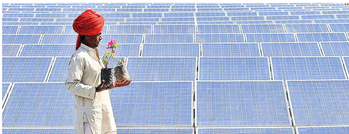
Image VII: Solar panel installations (NSM) (The Economic Times, 2020)
